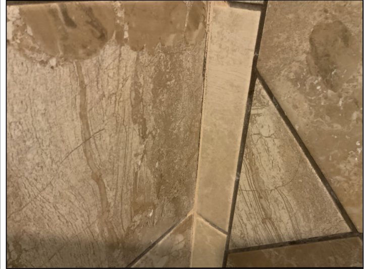
Missing grout noted at tile.
