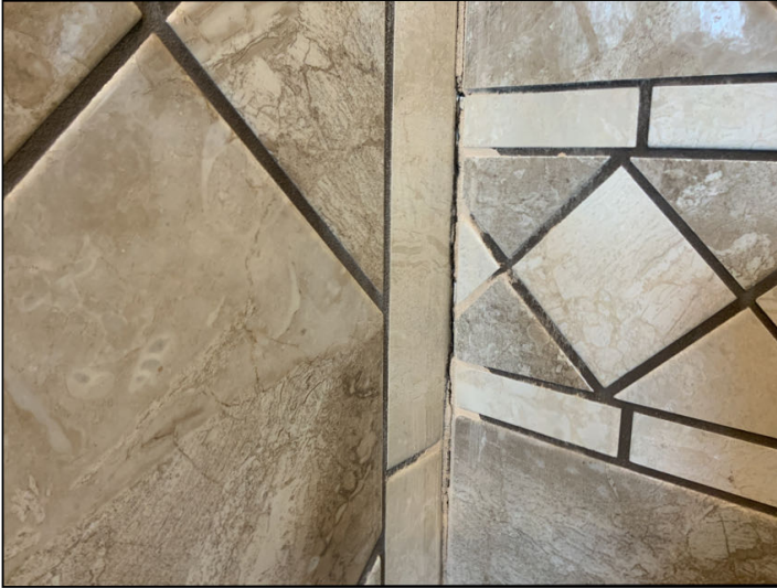
Recommend qualified contractor repair/replace missing/damaged grouting.
