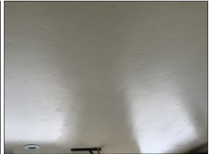
Evidence of past repairs.
