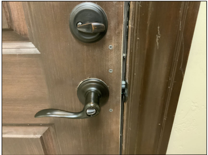
Screws present of both sides of door
