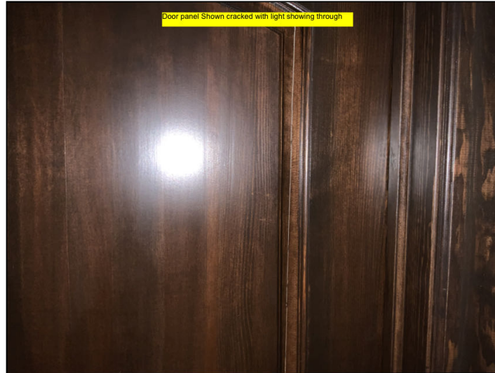
Door Cracked and damaged
