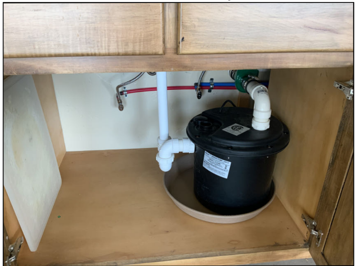
Garage has sink with undercounter pump/grinder for drainage
