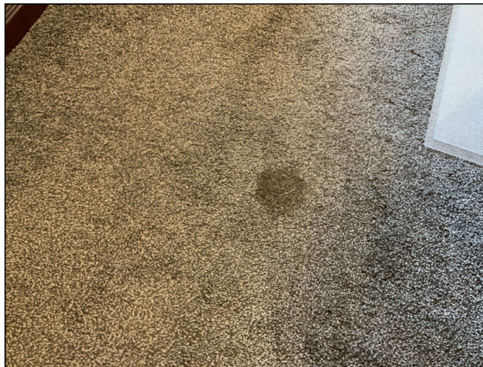
Typical stains and wear observed.
